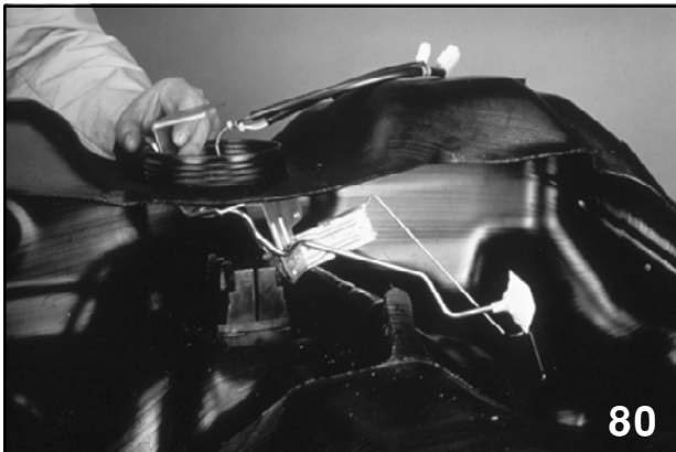
Removing Sending Unit
